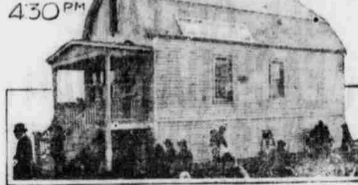
The Lumbermen's Association of Chicago, recently finished a five-room house in one working day. The foundation above was laid the day before. Building started at 8 o'clock. At 10:30 the house was half finished except, and at 4:30, quitting time, it was all ready to move into below except for the plastering.
