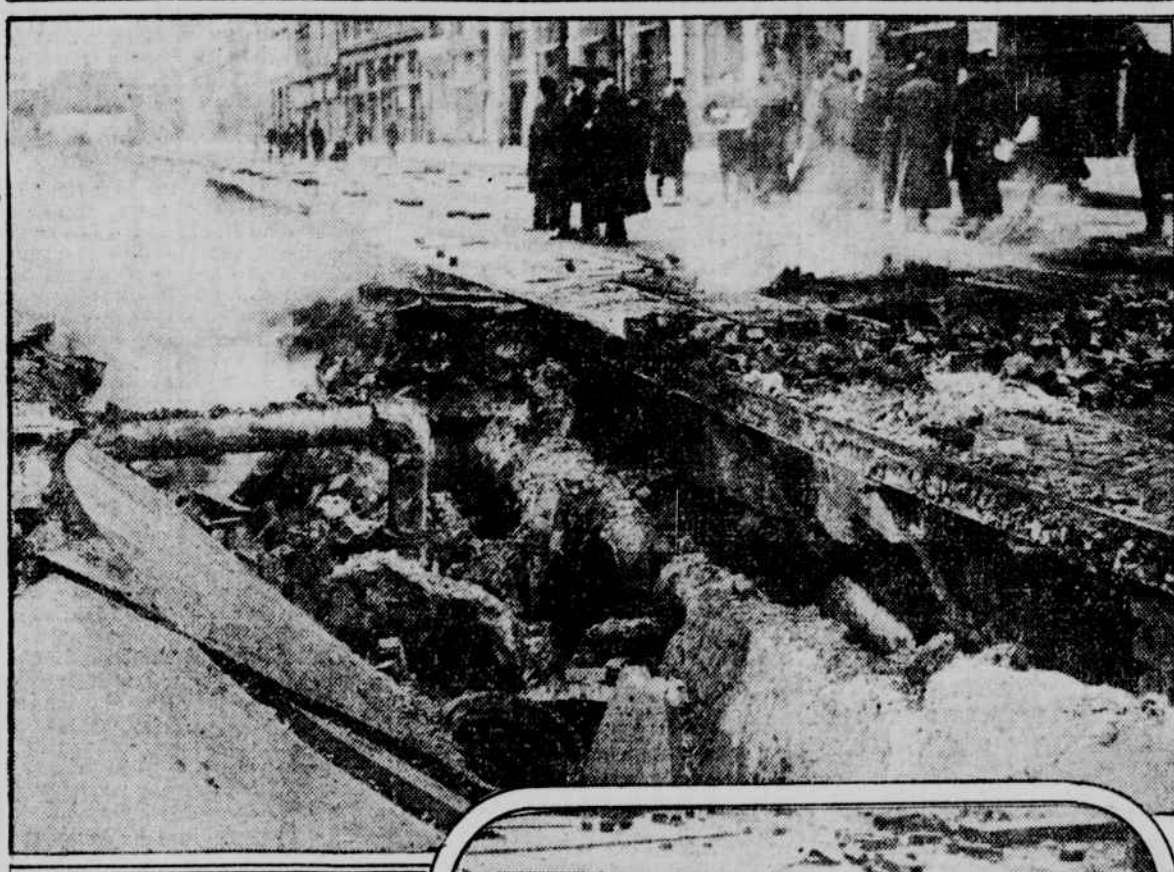
General scene at 23d street corner, showing how car tracks were left unimpaired.
