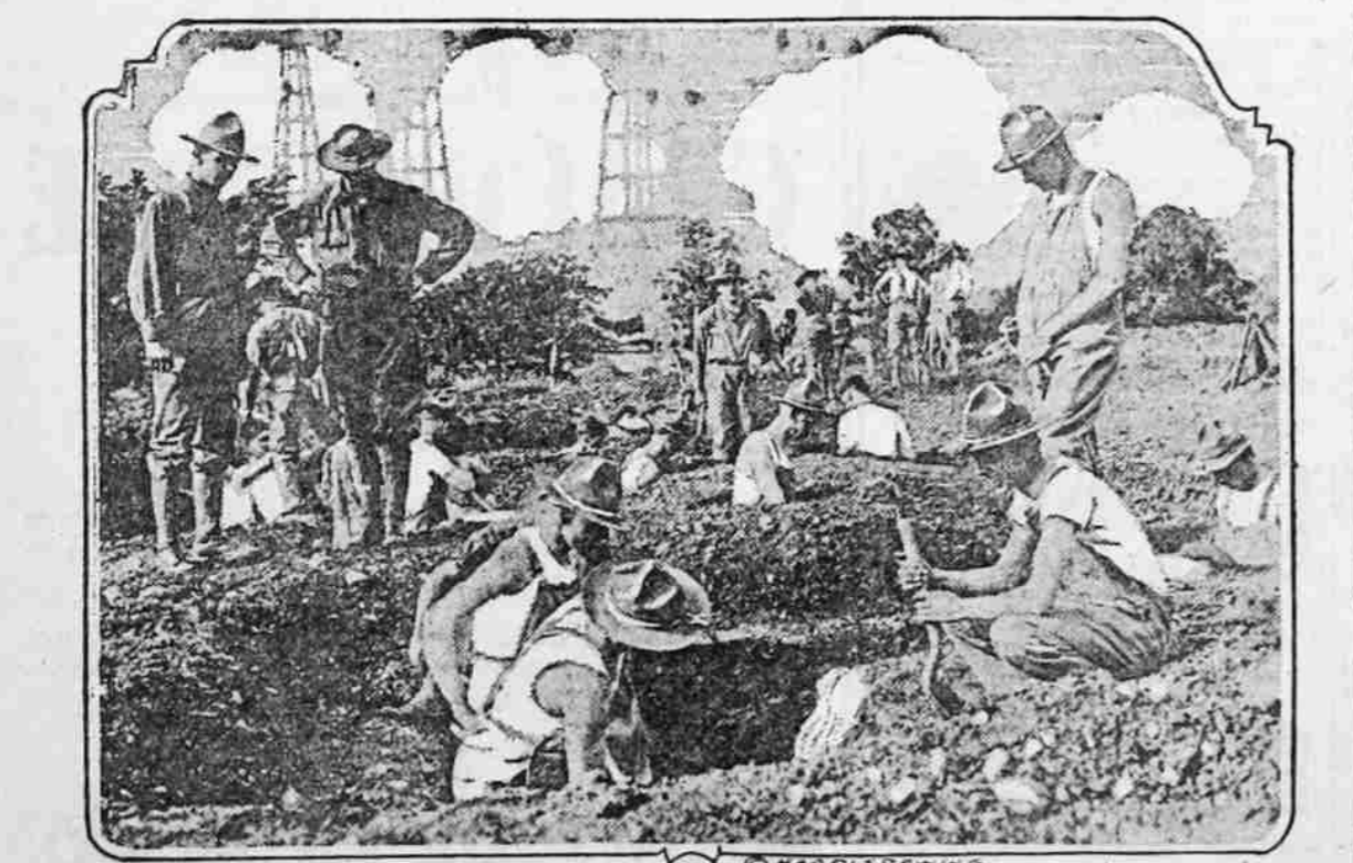
Digging trenches at officers' reserve camp, Fort Myer, Va. Young men of America's leading families who are training to be officers at Fort Myer, Va., are digging trenches, struggling with barb wire entanglements and erecting barricades as a part of their training for positions of command. These lads are digging trenches, not overseeing the job.
