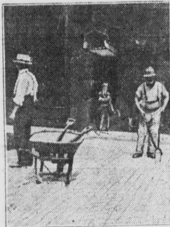
Granite Blocks Laid and Rammed — Maintenance Cost of This Kind of Pavement is Less Than That of Any Other Kind.
